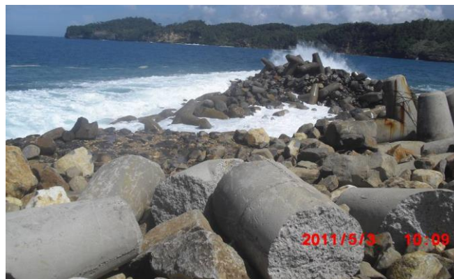
Figure 3. Rod Fracture of armour block on site
