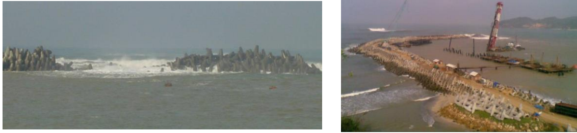
Figure 6. Site damage of section after the second repair
