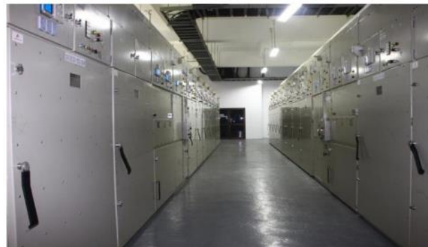
Figure 1. A physical example showing the external appearance of a 20 kV medium voltage switchgear (Source: PLN)
