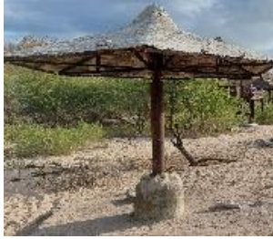
Figure 9. The condition of the gazebo in the Tablong Beach area
