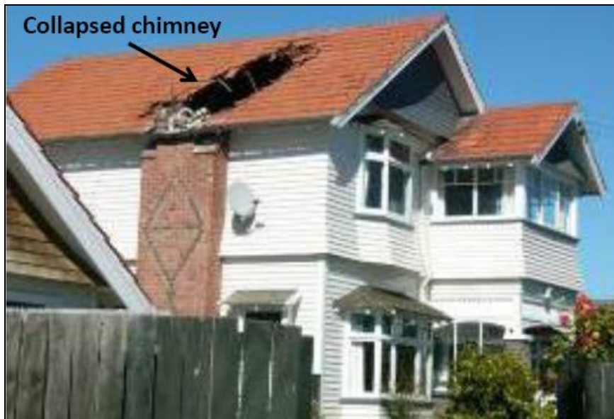
Fig. 5. Collapsed chimney of residential housing
