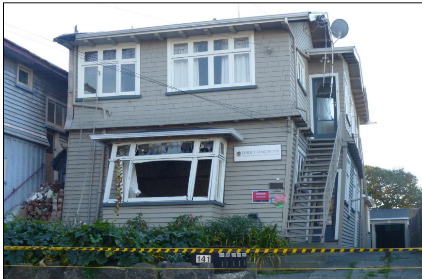
Fig. 6. Soft storey failure of timber housing
