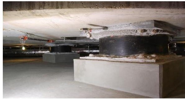
Figure 1 The seismic dampening widgets (Base Isolators) under the Utah State Capital building (Mike Renlund, 2008)
