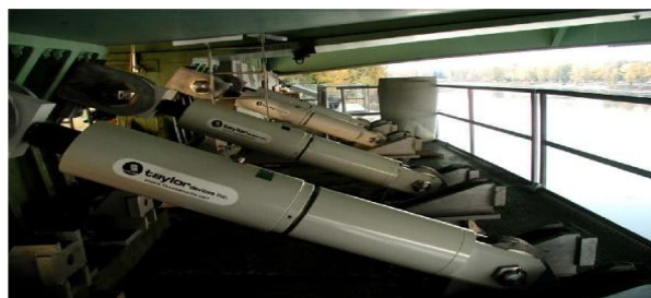
Figure 2 Fluid viscous damper system in a building (Taylor devices inc. annual report, 2024)
