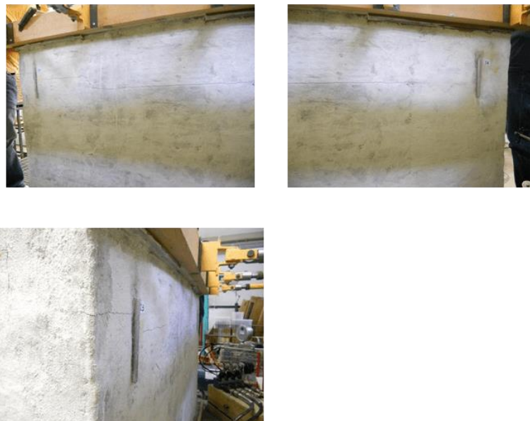
Figure 5 Damage of the unreinforced masonry house after one half cycle lateral loading in the experimental work [16].
