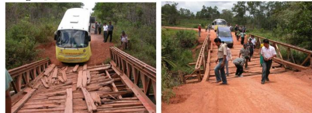
Figure 1 Condition of many small bridges in remote parts of Indonesia due to rapid deterioration of the bridge foundation[3]
