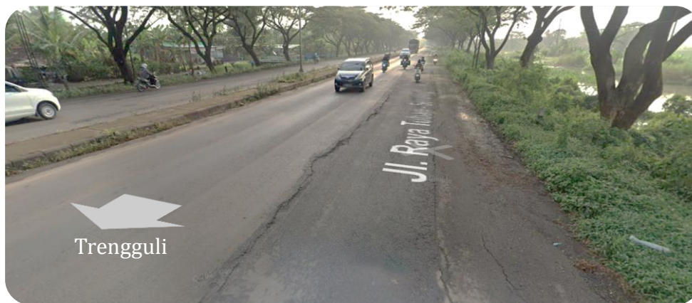
Figure 1. Road Damage on the Tregguli - Kudus Section KM 39+850
