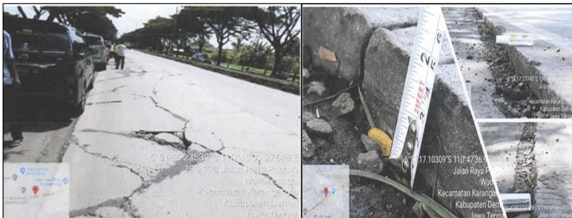
Figures 3. Road damage that occurs Source : BPLJ, 2021
