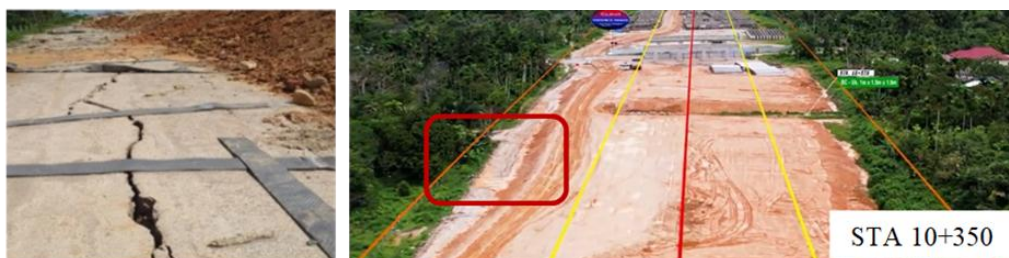
Figure 3. Cracks in the embankment toe STA 10+275-10+375 Line A (Sicincin-Padang Toll Road Project Team, Padang, 2023)
