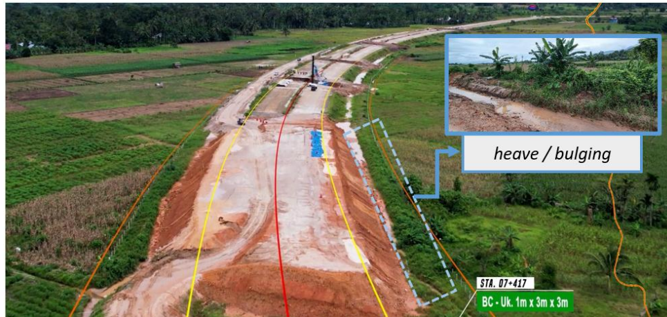
Figure 3. Heave at toe of embankment STA 7+450 R
