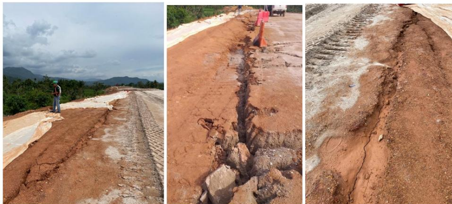
Figure 2. Cracks on the top surface of embankment STA 7+450 R
