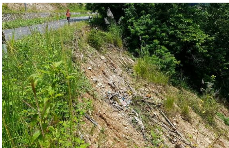
Figure 4. Cracks on the slope (PPK 2.1, 2019)
