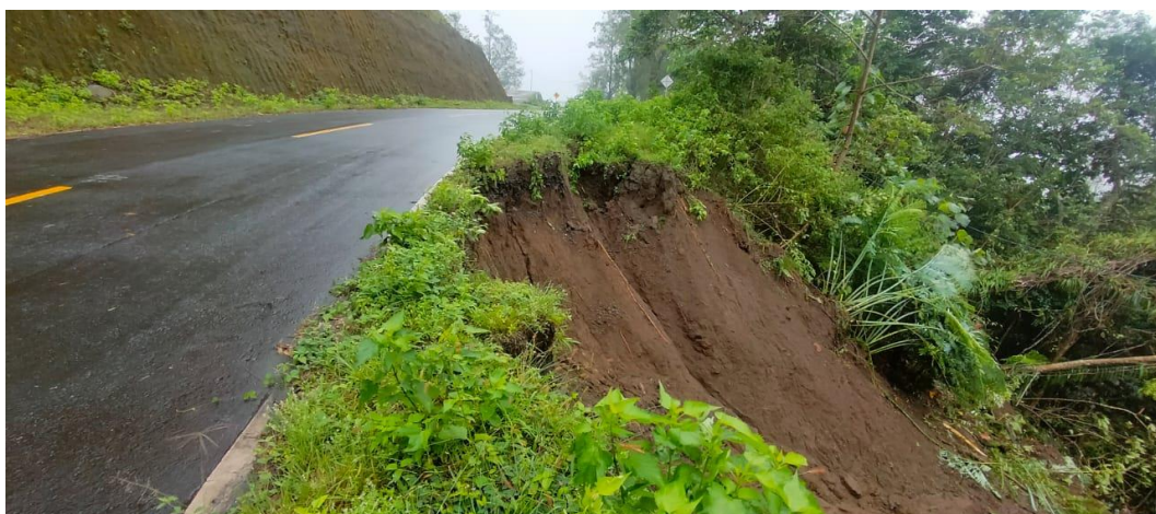
Figure 7. Landslide at STA 8+425
