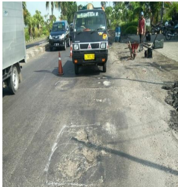
Figure 1. Road Damage On The Tuban–Babat–Lamongan–Gresik Road Section, Indonesia source: BBPJJN East Java – Bali, 2021
