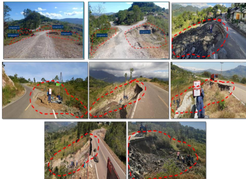
Figure 2. Sliding Slope on the Mota'ain-Motamasin Road Section
