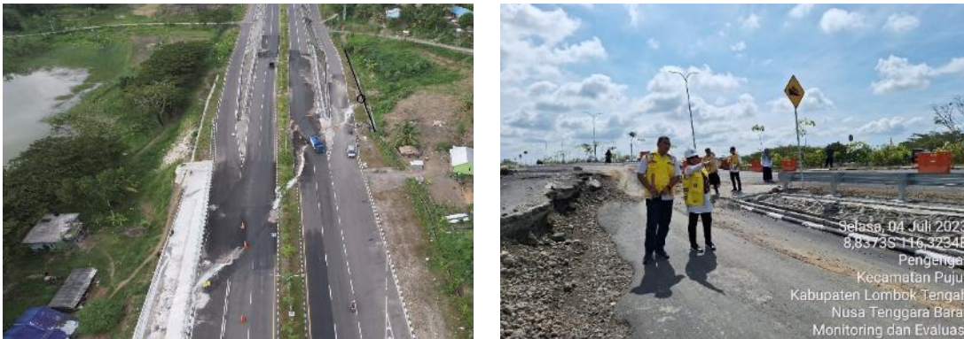
Figure 2. Landslide Surface on the road section Bypass BIL – Mandalika Km 10+415 s.d. Km 10+519 (Satker P2JN NTB, 2024)
