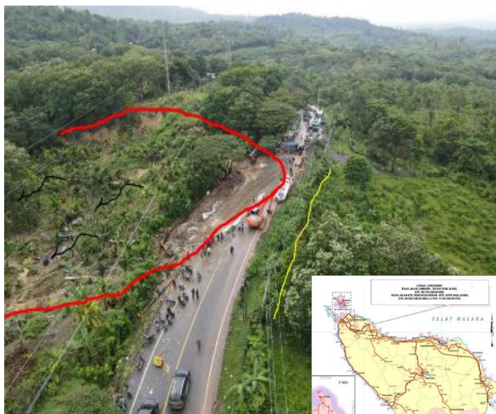
Figure 1. Landslide on the National Road Section of Batas Aceh Besar/Pidie - Batas Kota Sigli Sta. 0+500
