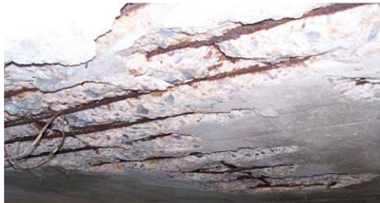
Figure 1. Corrosion in Reinforced Concrete Slab of Jetty Structure
