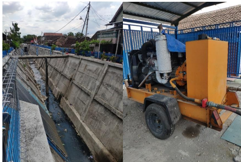
Figure 2. Channel (left) and Mobile Pump (right) in Pancasila pumping station
