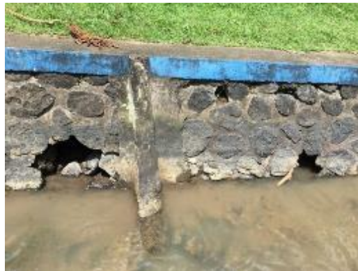
Picture 6. Channel Wall Damage Due to Erosion
