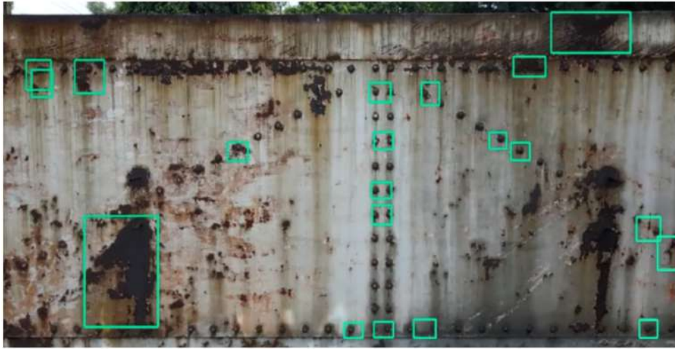
Figure 6. The result of corrosion detection using CNN.
