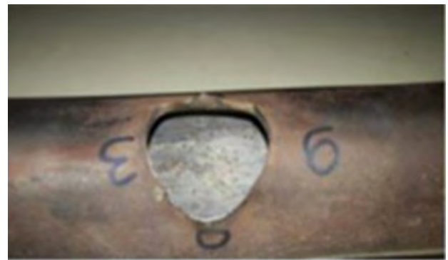
(b) The oxide layer failure characteristics tube with tube code 7
