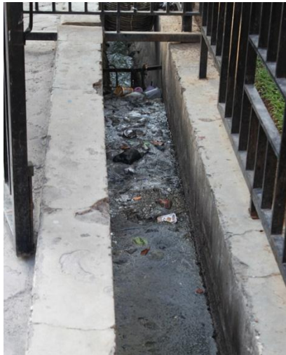
Figure 5. Drainage Conditions In Sombo Flats (Source: survey results, 2012)
