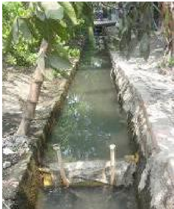
Figure 6. Drainage System in Desa Sadang
