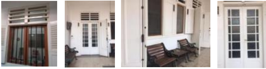
Figure 26. Existing doors and windows of the house of Mr. Isaac Source: personal documentation
