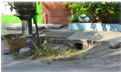
c. Provision of bins to reduce waste buildup burden on drainage.
