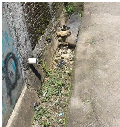
Figure 9. Example of Inadequate Drainage Condition in the Settlement Area Source: field survey, 2014
