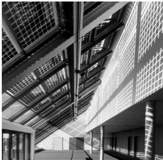
Figure 2. PV Panel Installation at Public Building with Optimum Tilt Angle and Fixed Orientation Source: Benemann, dkk, 2001
