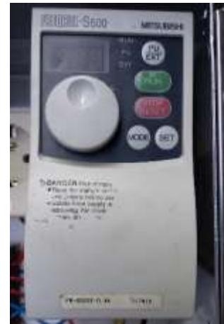
Figure 3. Variable Frequency Drive for SLC Plant
