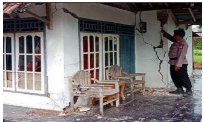
Figure 3. Types of Damage to Residential Houses After the Earthquake Category Light Damage (Source : Survey, 2022)
