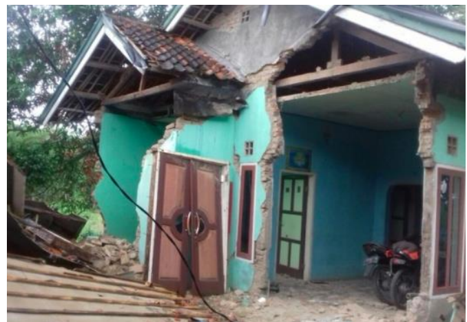
Figure 2. Types of Damage to Residential Houses After the Earthquake Category Medium Damage (Source : Survey, 2022)
