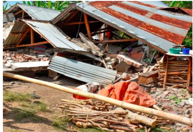
Figure 1. Types of Damage to Residential Houses After the Earthquake Category Heavy Damage (Source : Survey, 2022)
