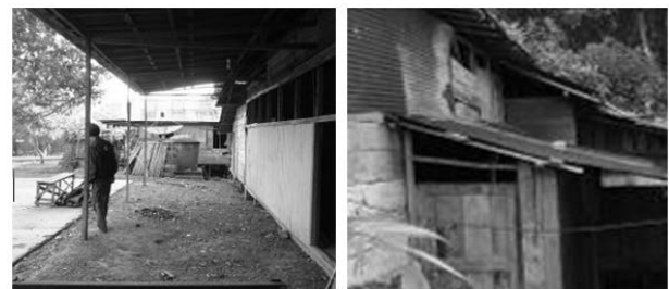
Figure 9. Overhang Condition. Long Overhang in Front of Building at Laras-Pematang Room (Left) and Short Overhang in Left, Right and Behind of Building at Bilik Rooms (Right)
