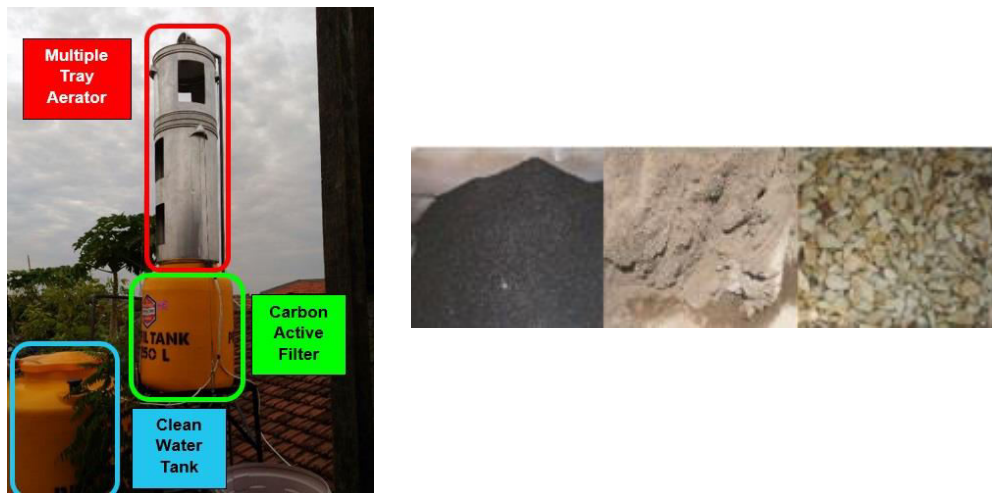
Figure 2. (a) Water Treatment Unit Installed on Site (b) Media Used in Filter Unit
