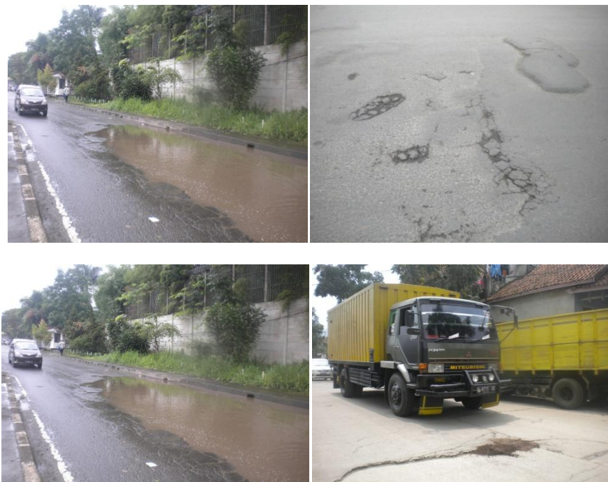
Figure 2 Left: Water ponds in MM and K street, Right: Pavement distress in MM and K street
