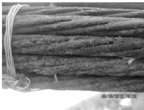
Figure 4. Myaungmya Bridge Main Cable Damage
