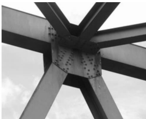
Figure 2. Rust Panel Point of the Truss (Bomyatun Bridge)
