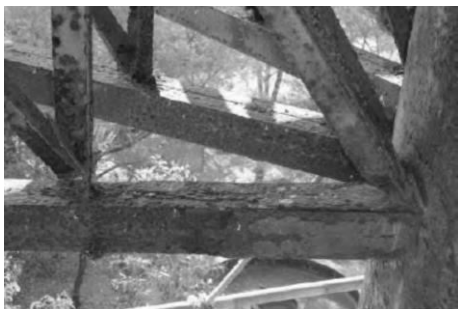
Figure 3. Myaungmya Bridge Corrosion
