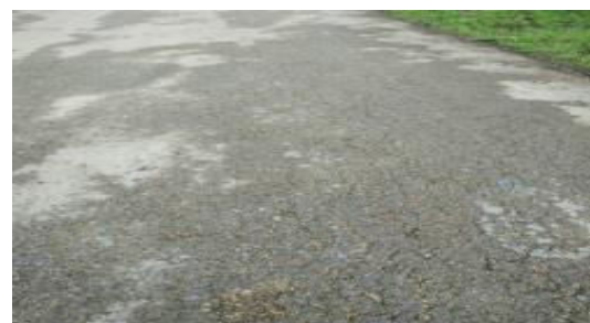
Figure 3.2c. Type weathering damage and raveling With a high degree of damage to the Biak-Korem-Supiori road
