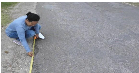
Figure 3.1b. Type of crack fracture edge with moderate damage level on Aminweri-Yendoker road
