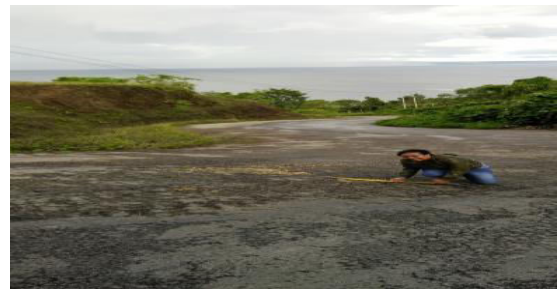
Figure 3.1c. Type weathering damage and raveling With high damage levels on the Aminweri-Yendoker road
