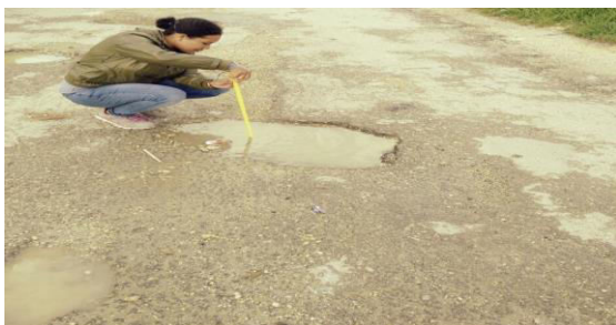
Figure 3.1a. Type of hole damage with high damage level on Aminweri-Yendoker road
