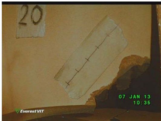
Figure 4. Missing Trailing Edge
