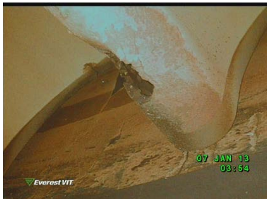
Figure 5. Hole at Leading Edge
