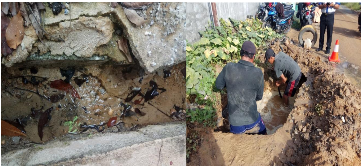
Figure 5. Leaks in house connections and Pipe Distribution Network
