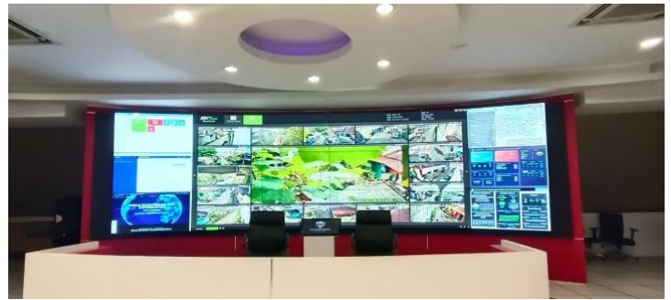
Figure 2 CCTV Control Room in Makassar City
