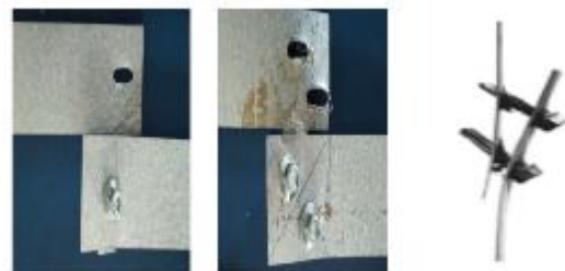
Figure 7. Failure mode of screw connections on the CFS structure
